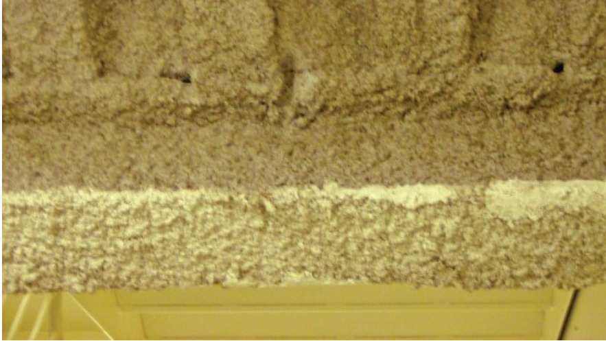
This beam was covered in fireproofing material in an example of passive fire protection.
